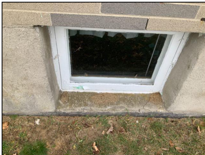
2. Paint or stain needed
