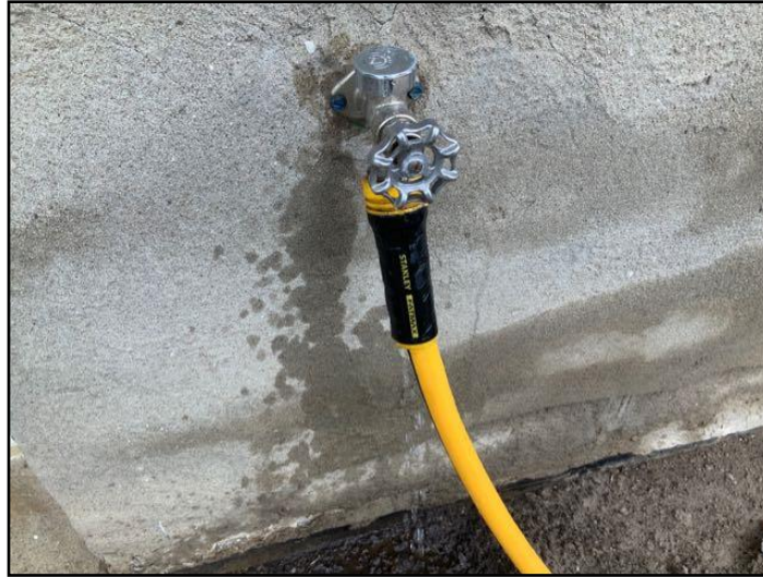
23. Leak or drip
