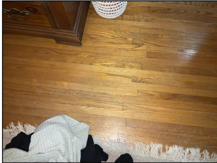
27. Various areas of the flooring was worn. To...
