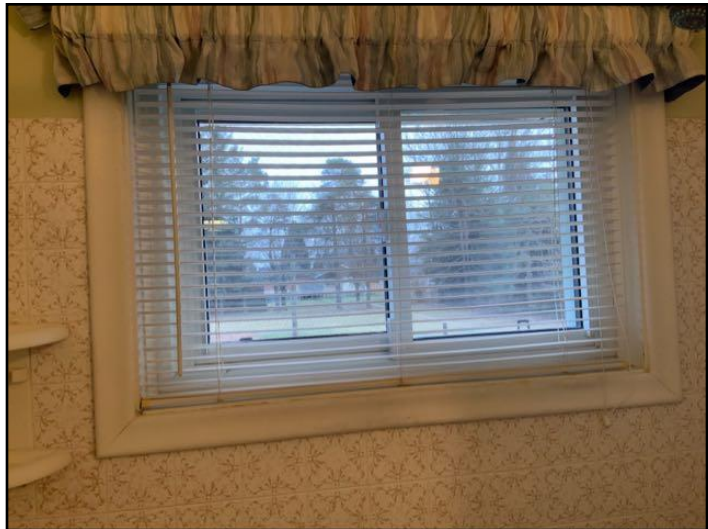
24. The bathroom of the home has an unprotected...
