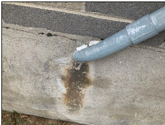
1. Caulking missing or ineffective
