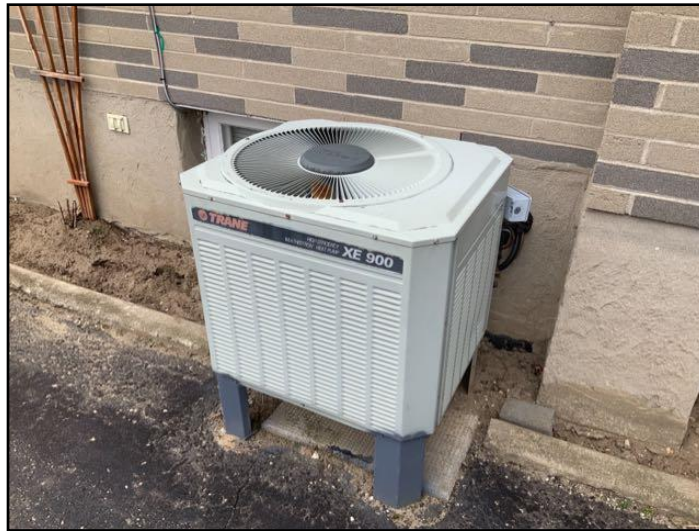
18. Service air conditioner
