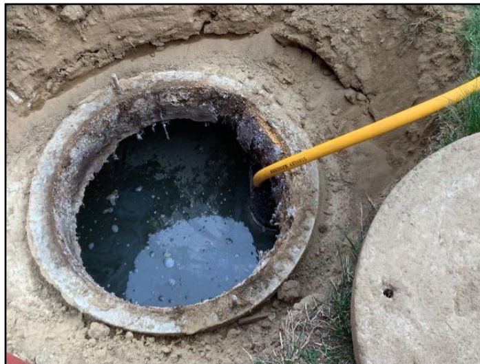
31. It is recommended to have an effluent filte...
