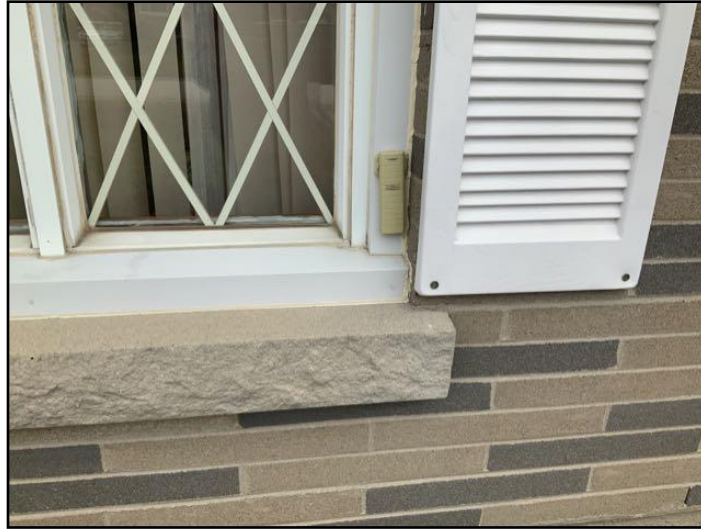
3. Caulking loose, missing or deteriorated
